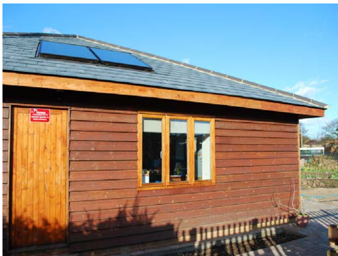
Solar thermal panels on the 'Growing Together Community Garden' project in Prittlewell Chase.
